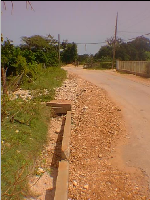
Photo 5 U-drain blocked with marl preventing free conveyance along Great Bay parochial road
